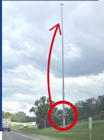
HIGH MAST LIGHTING
