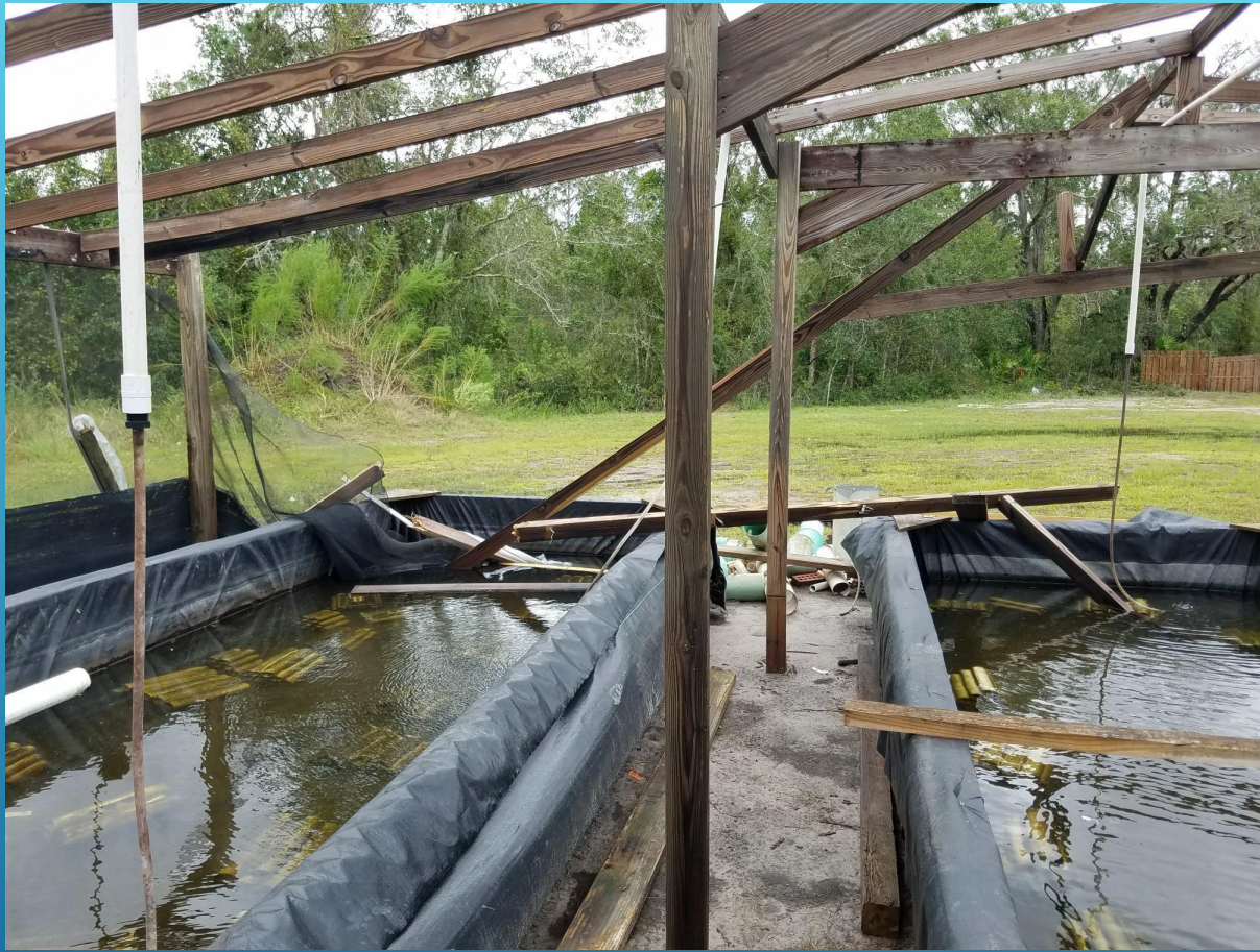
Wind damage to screen structure, St. John County
