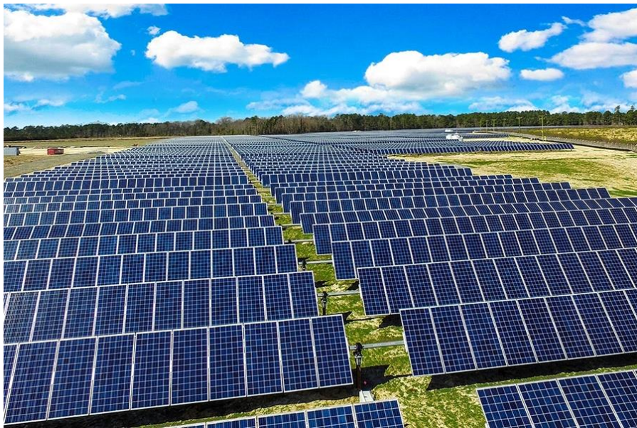
(Image of Photovoltaic Panels) 28
