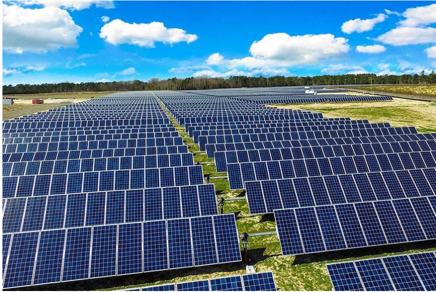
(Image of Photovoltaic Panels) 28
