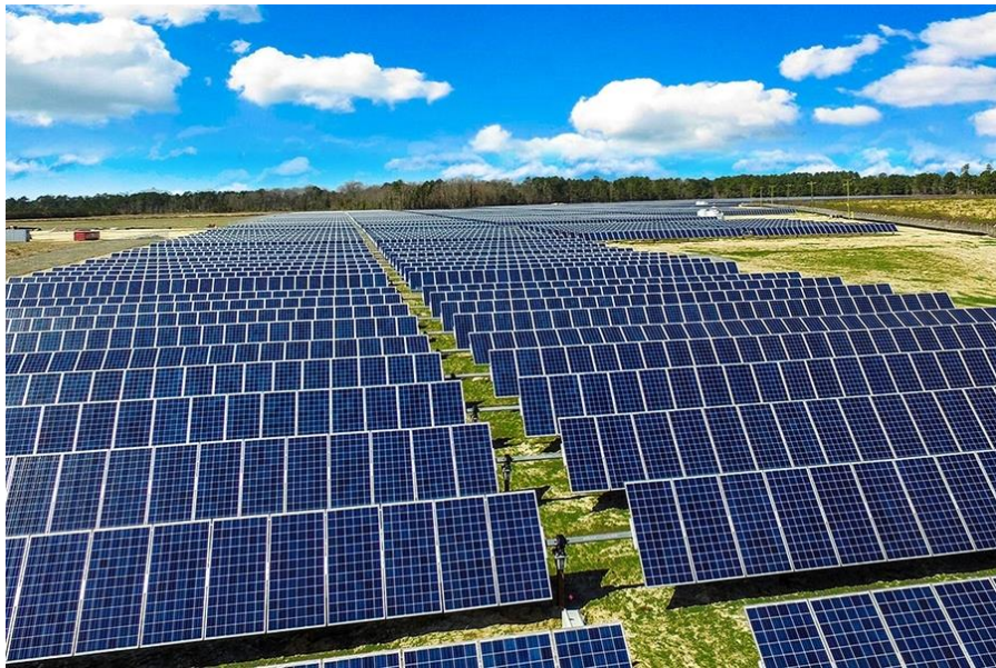
(Image of Photovoltaic Panels) 28
